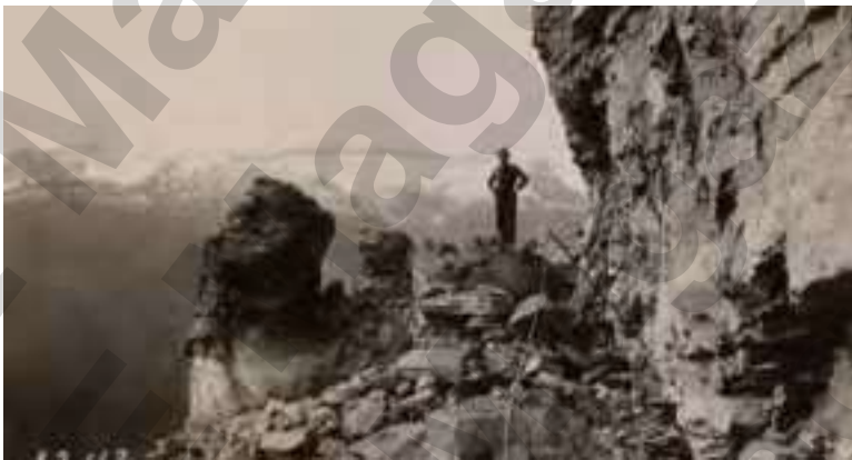
Top: Photo taken in August 1926 "Showing car and track method of handling excavation by stationmen. Garden Wall and trail on left. Logan Pass in middle background." From: Final Construction Report for Transmountain Highway (1928) by W. G. Peters U.S. Bureau of Public Roads Photo courtesy of the Glacier National Park Archives
